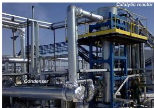
Reactor with fluidized bed of catalyst
